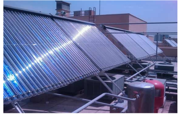
Figure (2) – Solar heat pipe system in 3th Khordad building in Tehran.
