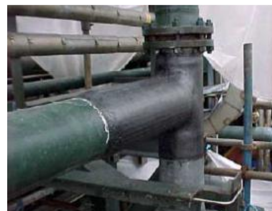
Figure 2. Carbon fibre repair of 14 inch tee joint on a seawater return header
