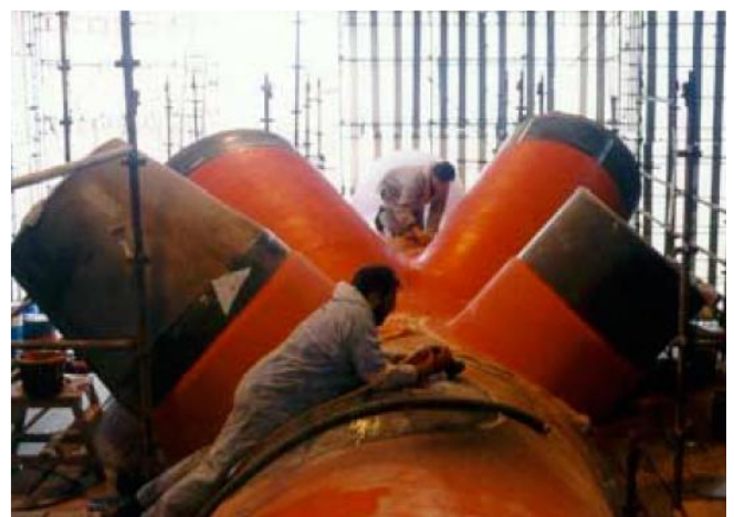
Figure 3. Composite combined corrosion and fire protection being applied to a steel tubular
